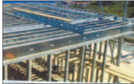
STEEL FRAMING PROVES a viable plan for construction in many different climates, according to a recent study.
